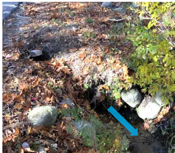
6: Drainage pipe on Pleasant Valley Road
