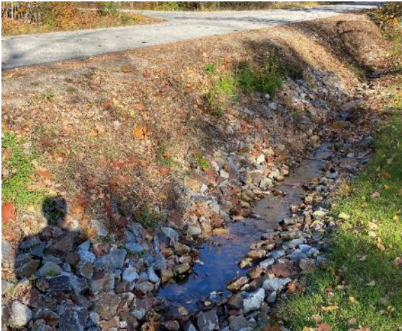
Photo 4: Minor erosion observed at edge of road /top of slope to drainage channel
