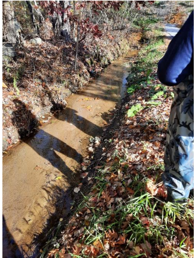
Photo 8: Significant accumulation of sediment from stormwater runoff in channel
