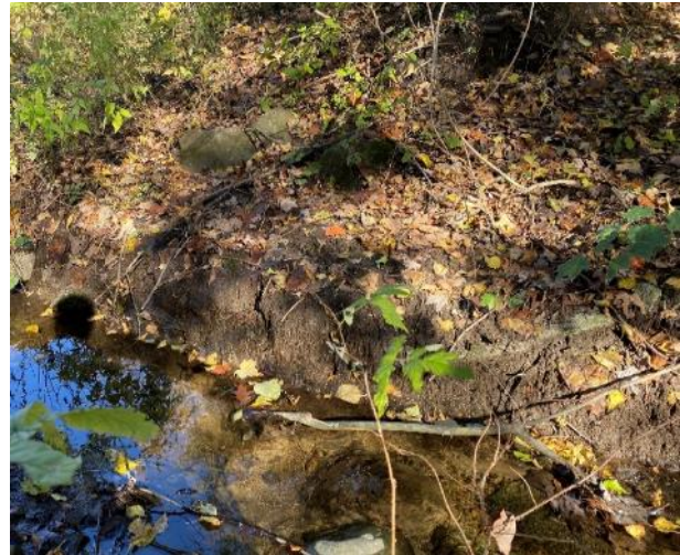
Photo 15: Minor bank erosion
