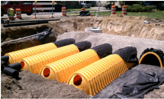
Installation of a subsurface infiltration basin to manage stormwater runoff from a large
