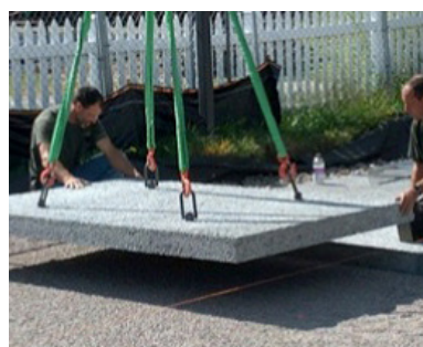
A pre-cast permeable concrete parking lot being laid on the UVM campus in Burlington.
