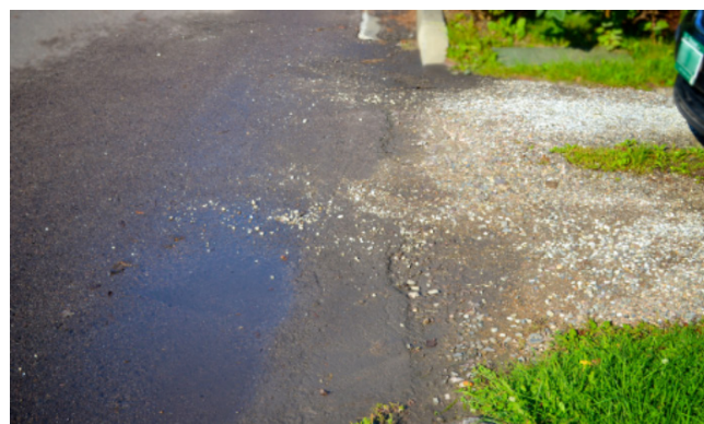
A gravel driveway without proper slope and drainage. Gravel and oils are washing into the street.
